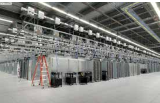
▲ One of Google's servers. Google has 16 server locations around the world. These mammoth facilities hold your personal data.
